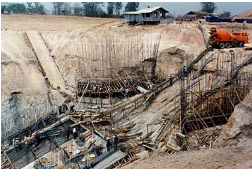
Fig.4 Demonstration of mass concreting using fly ash concrete at Mae Moh power generating plant
