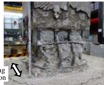
(b) After removing CF-panel and crushed concrete
