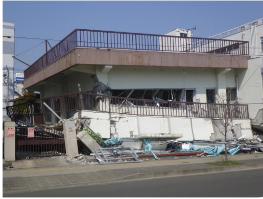
Figure 2 Reinforced concrete building collapsed by the earthquake in Sendai
