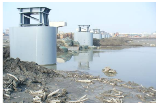
(Fig. 13) Adding 2 M high formed steel structure on top of pier and the RC piers are clad with steel plate and constrained with concrete.
