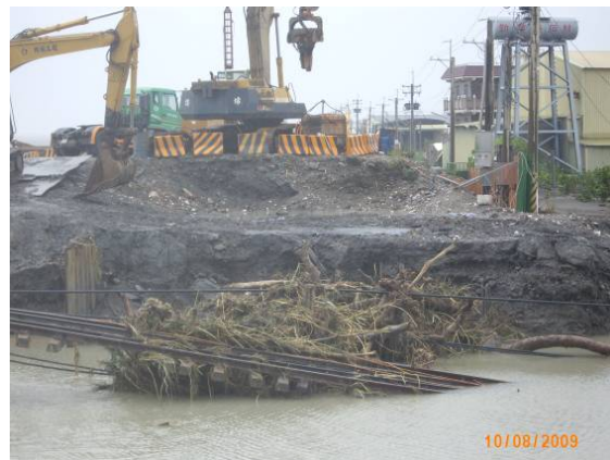
(Fig.10) Damages to north abutment 、Washed off Road Base.
