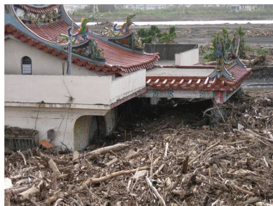
(Fig. 6) The water level is as high as to the 2 nd floor and muddy water is flowing everywhere.
