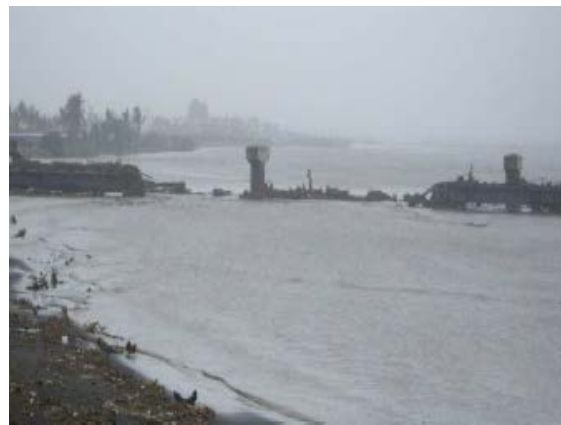
(Fig. 9) Washed off 2 piers and 3 spans (P10/11/12)
