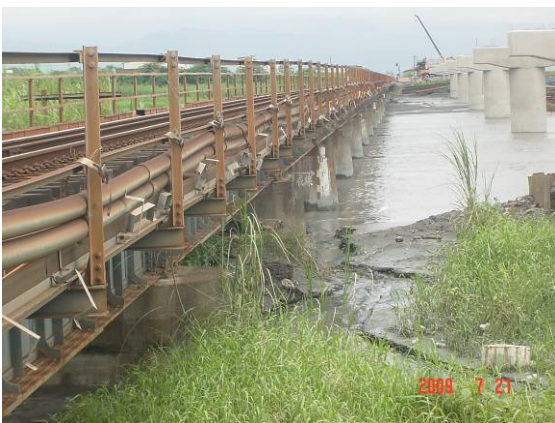
(Fig. 5) Bridge Pier of New Linbian River Bridge at the downstream side of old bridge.
