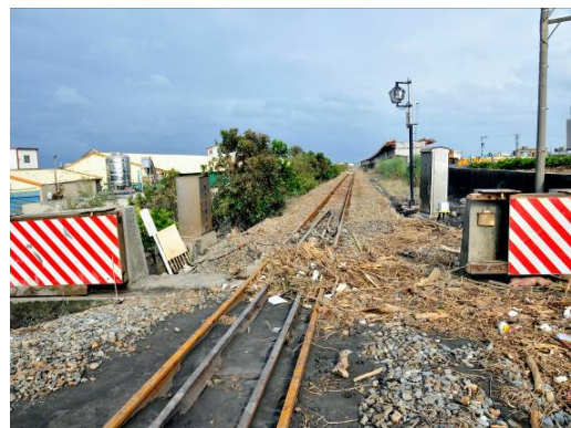
(Fig. 16) South side gate was intact after the disaster due to deposit and stacking of drifting articles brought by the flood.
