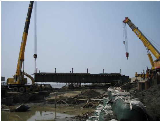
(Fig. 11) Bridge Steel Beams are totally lifted and moved away from site
