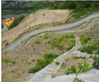
Fig2.6 Completed lateral and longitudinal drainage project on landslide scar at 5K on Tengzhi Forest Road.
