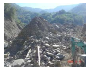
Fig2.1 Before removal of sediment from Toukeng Creek in Xinyi Township, Nantou County
