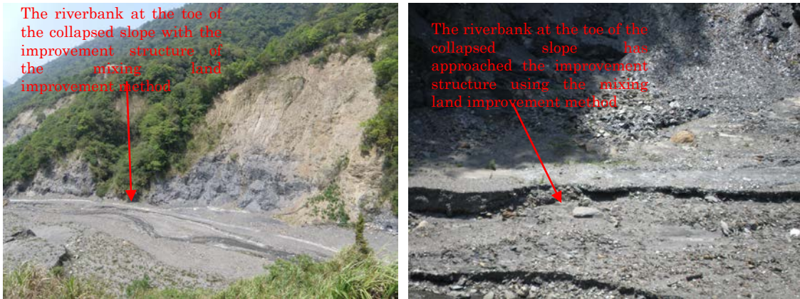
Figure 4-3 Hewang mixing land improvement engineering method used to protect against collapsed land
