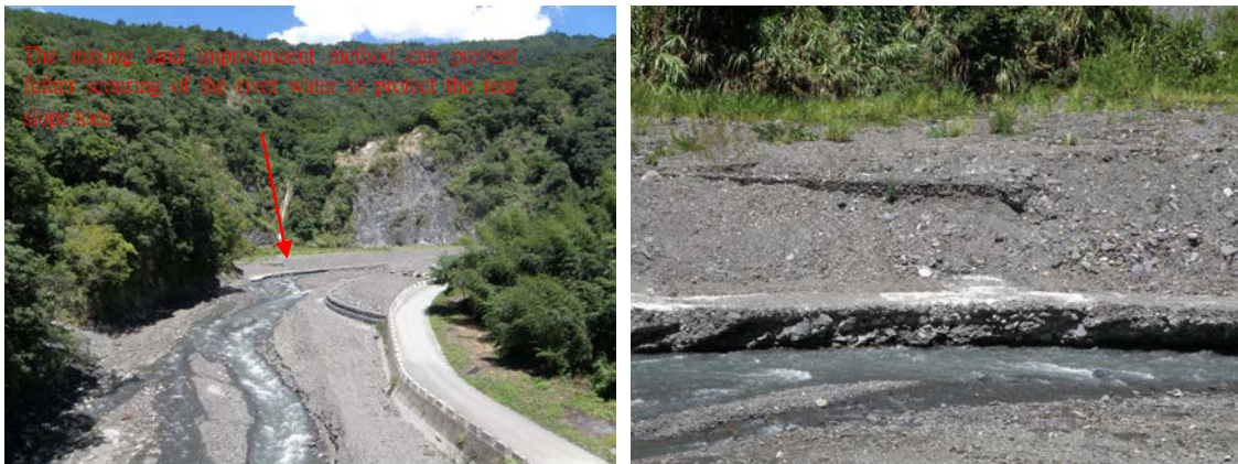
Figure 4-4 Honghsiang mixing land improvement engineering method used to protect against collapsed land
