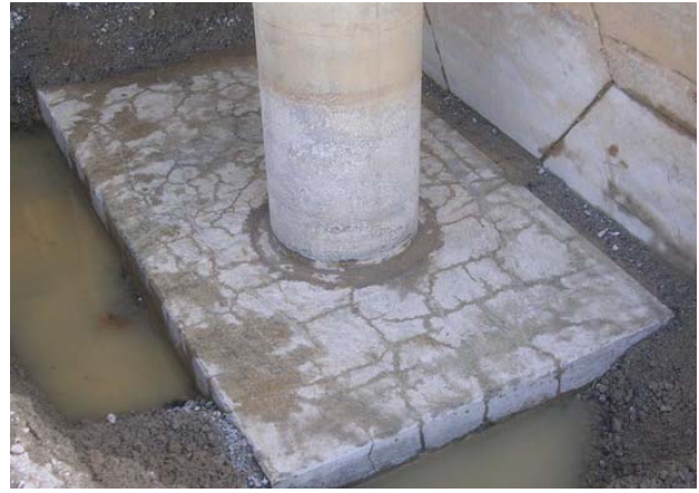
Figure1 Map cracking in a pile cap
