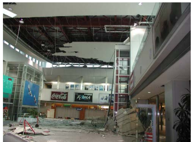
Figure 2 Ceiling of the airport terminal fell down by the Off Tokachi Earthquake in 2003
