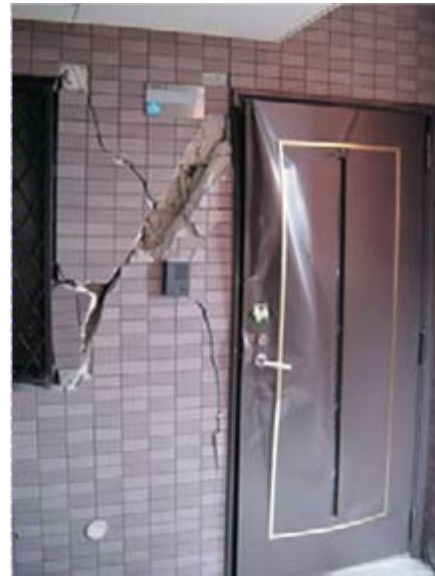
(b) Damage of the non- structural wall and door
