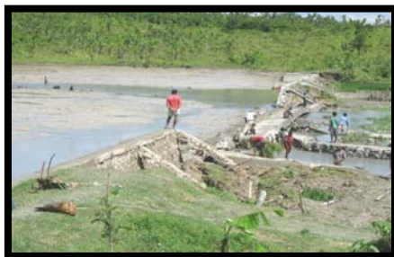
Figure 7. Keruk Situ after collapsed.
