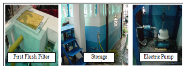
Fig. 2 Example of RWH installation in Selangor – separate system
