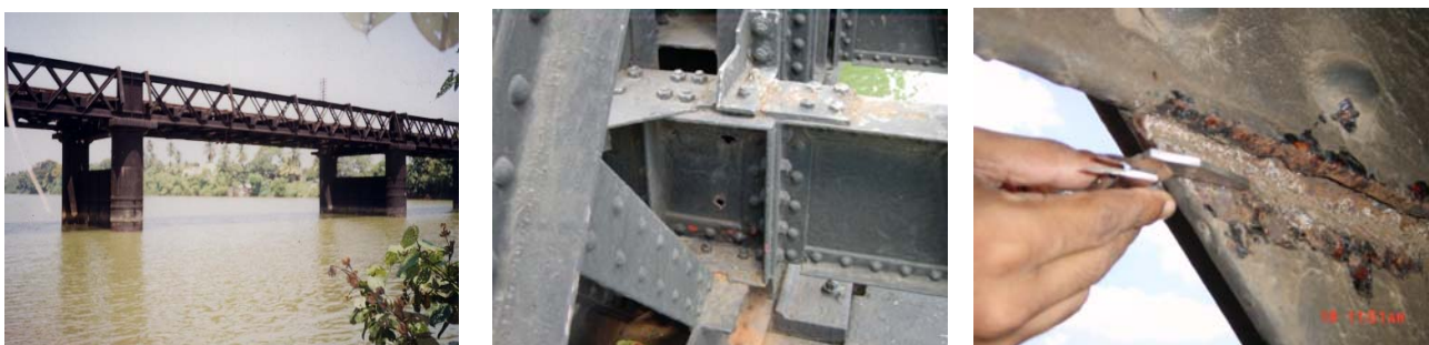
Fig. 3 General view and identified corroded locations of the bridge
