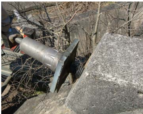
Picture 2. Degradation in anchor
