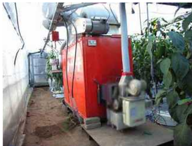
Picture 2 Wood-pellet burner attached to the heater
