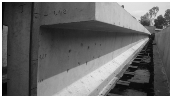
Figure 9: Pre-stressed T-girder with heavy flange, span 20 m, casted with high strength self-compacting concrete in Phnom Penh, Cambodia; Source: Vong, S. and Prof. Shima, H., KUT, Japan
